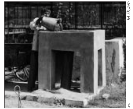
Figure 2: Brick masonry hopper for feeding fresh cattle dung into the plant
